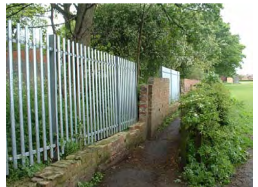
Fig. 33 Damaged sections of the northern boundary wall.
