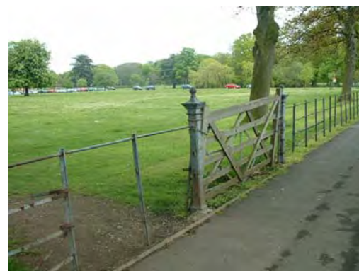
Fig. 35 Missing sections of fencing along Hall Drive
